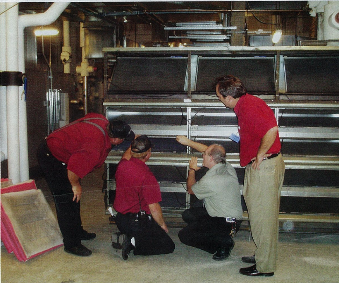
Sam's Town upgraded to electronic polarized-media air cleaners and extended their maintenance schedule more than twofold. Media is changed every six months, where previously the filters required changing every two to three months.
