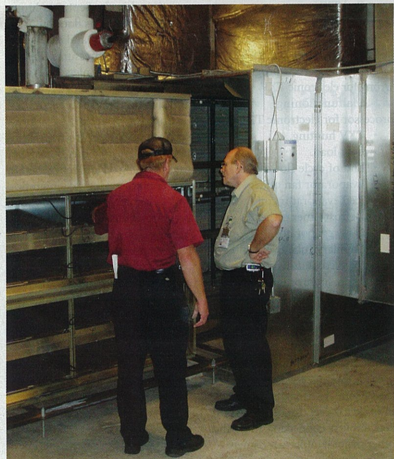
A Sam's Town HVAC technician and director of facilities Steve Richey look at prefilters on the air cleaner section in one of 12 air handling units at Sam's Town Resort & Casino in Tunica, Miss.
